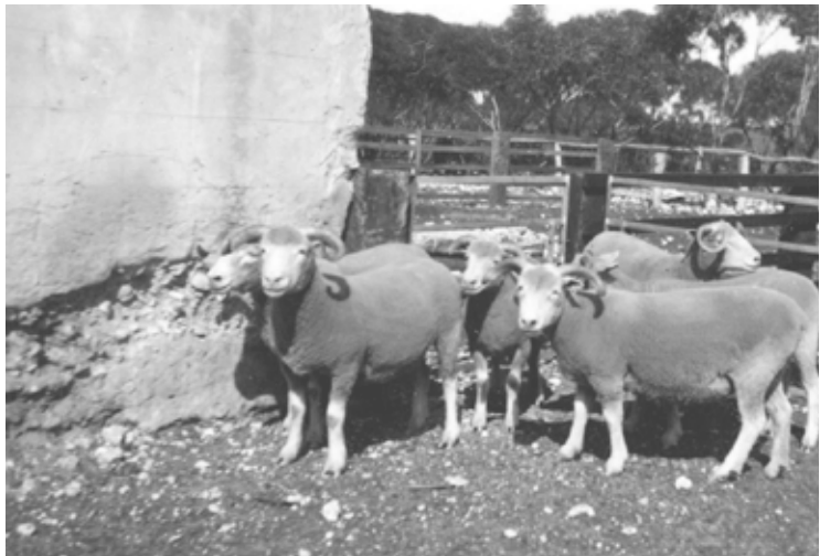
SALT DAMP ERODING AWAY THE ORIGINAL SHEARING SHED
